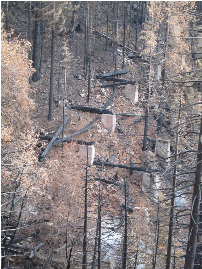
Trestle after fire.
